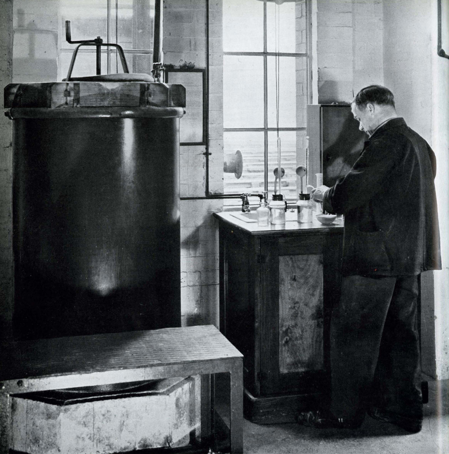
Testing bench on a typical Lime-Soda plant (Sodium Aluminate dissolving tank on the left).
